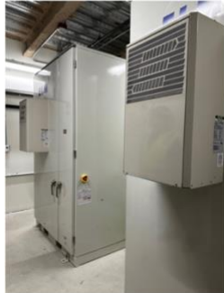
Battery system at the Kenzi
